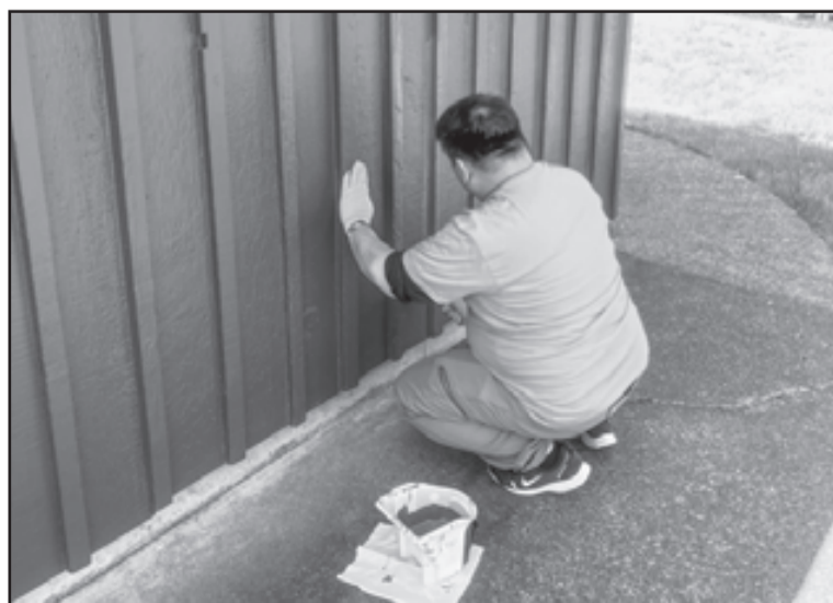
CC Rewell Encina ensures that the house's wooden siding is covered from top to bottom with a fresh coat of paint.
