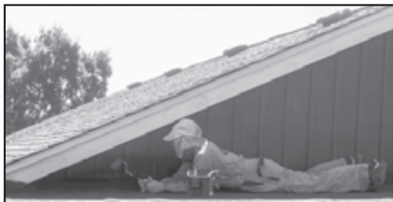
AB Len Soriano pays close attention to detail, repainting the trim on the inner corner of the roof.
